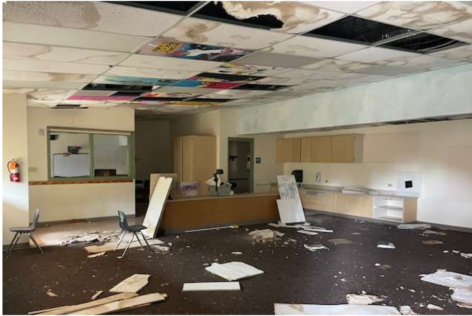
Subject interior – note ceiling damage
