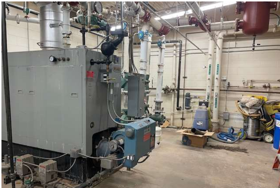
Subject mechanical room
