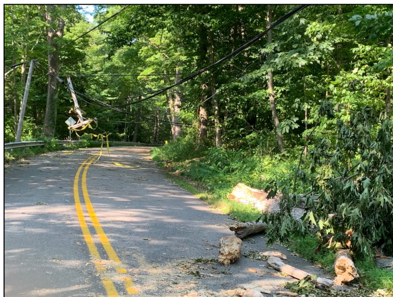
Damage from Tropical Storm ISAIAS on August 5, 2020
