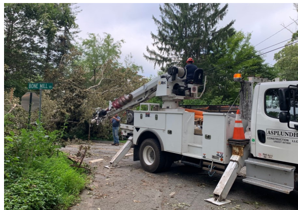
Damage from Tropical Storm ISAIAS on August 5, 2020
